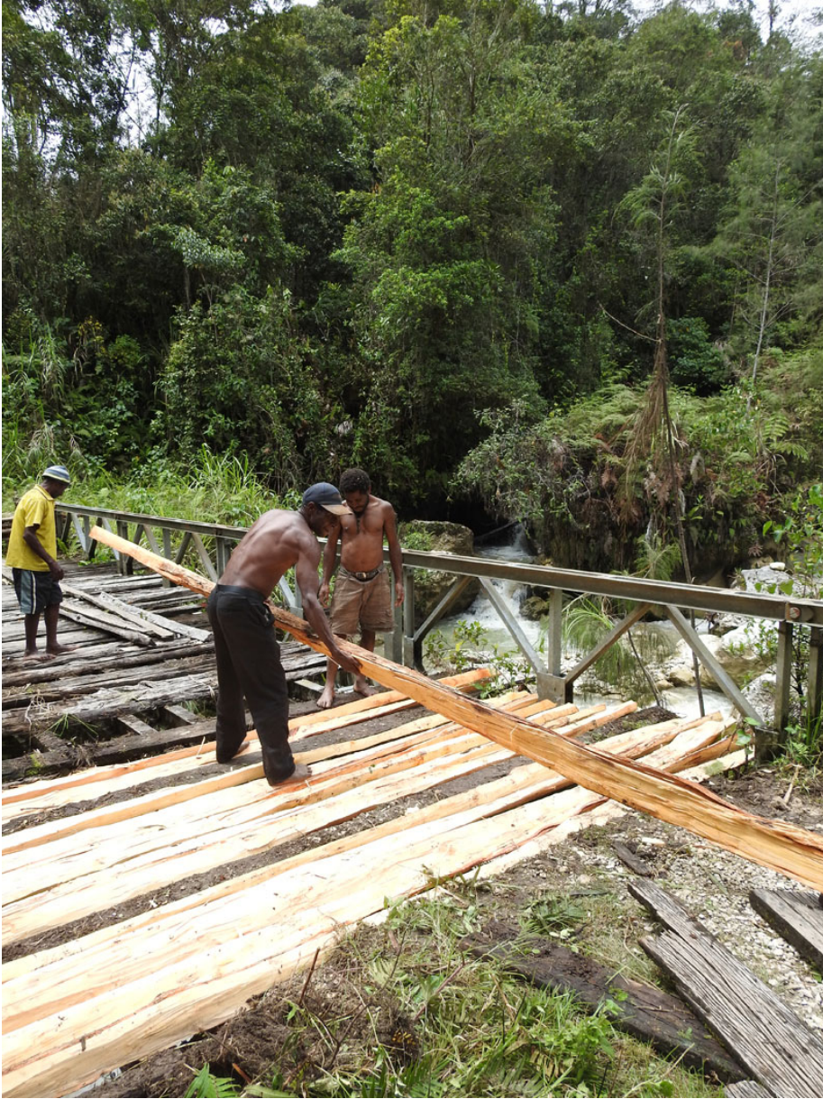
Figure 5 Bridge being repaired in eastern Porgera Valley. [Colour figure can be viewed at wileyonlinelibrary.com ]
