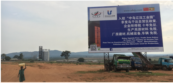
A China-funded industrial park under construction in Uganda; photo by Robert Wyrod
