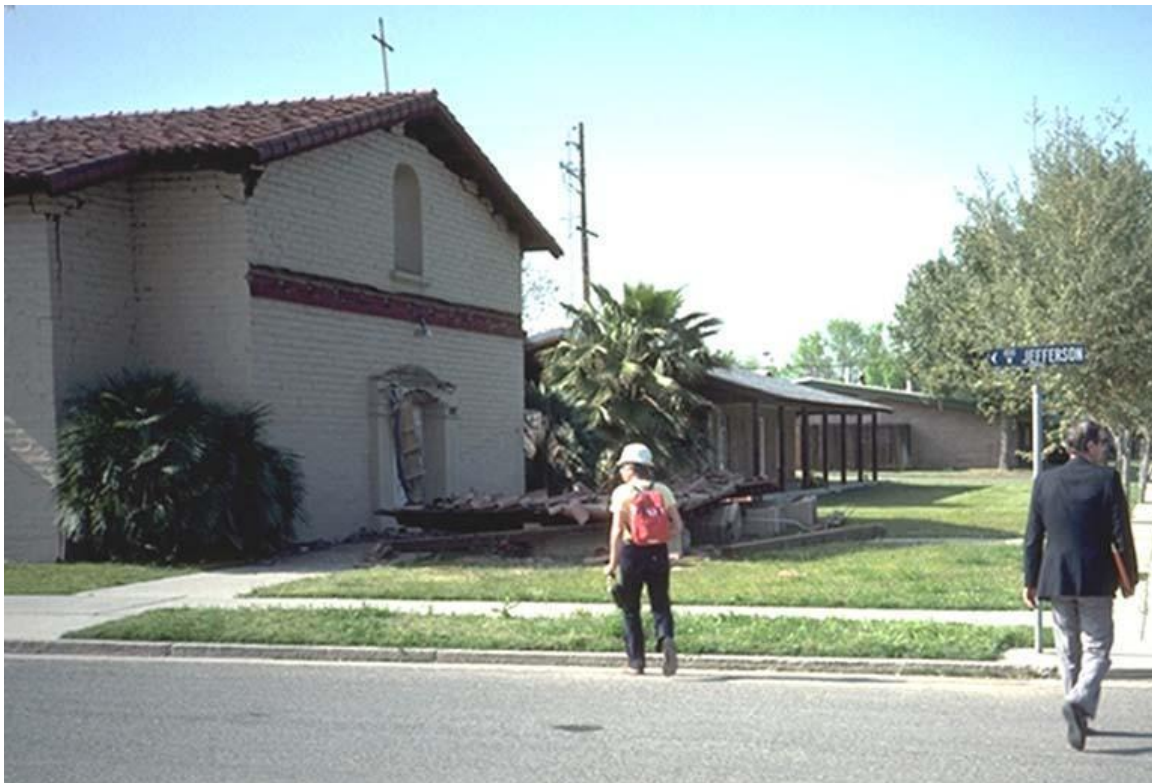
Figure 5–6. Image showing porch pulled away from church building in the 1983 Coalinga, California, earthquake.
