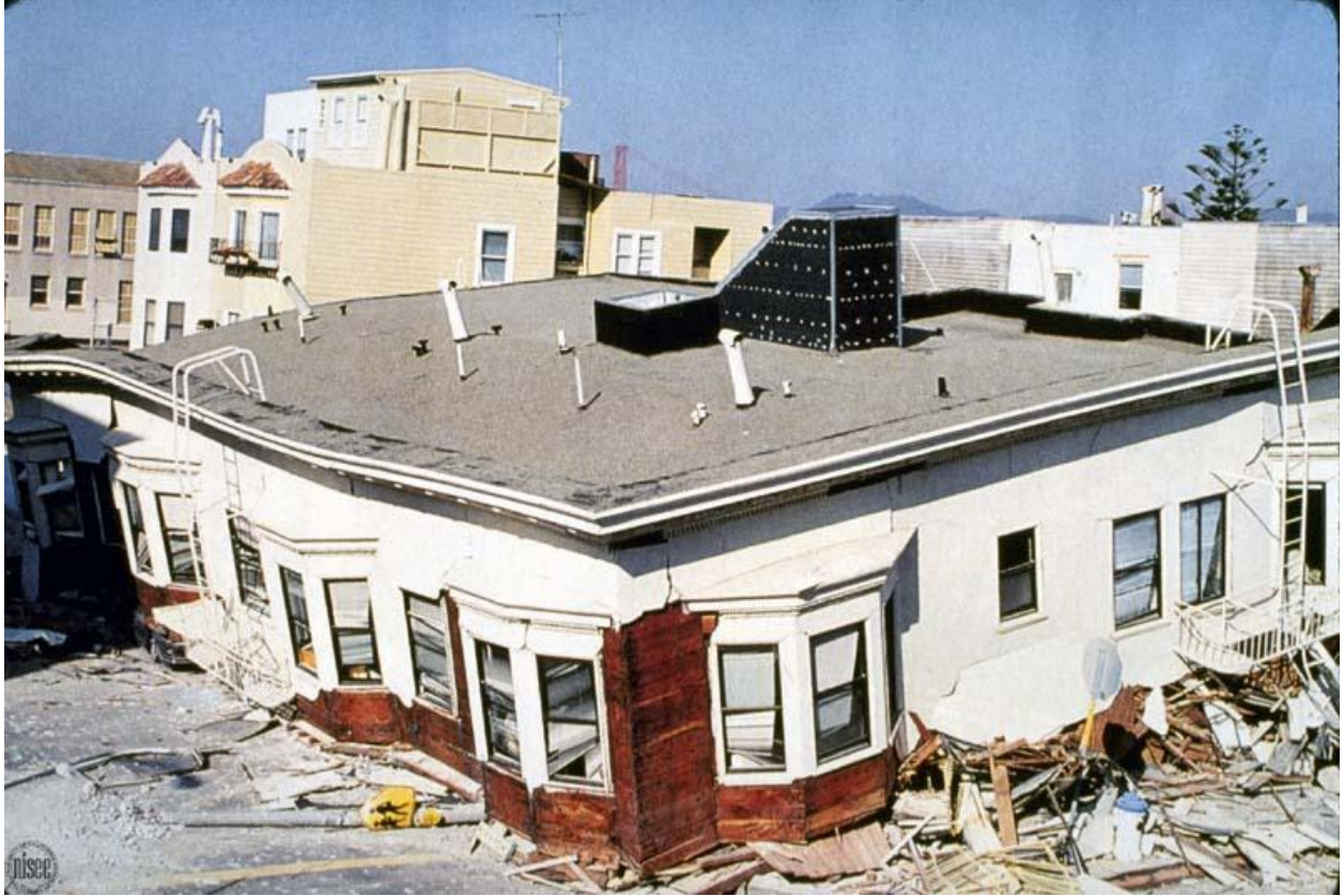
Figure 8–12. Image showing soft-story collapse of an apartment building in the Marina District, San Francisco, in the 1989 Loma Prieta, California, earthquake. Karl V. Steinbrugge Collection: S6144, copyright restricted.
