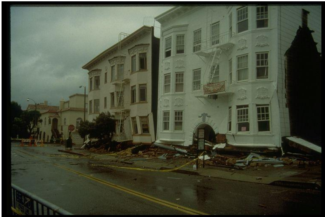
Figure 8–10. Image showing collapse of apartment buildings with soft ground floors in the Marina District of San Francisco in the 1989 Loma Prieta, California, earthquake.
