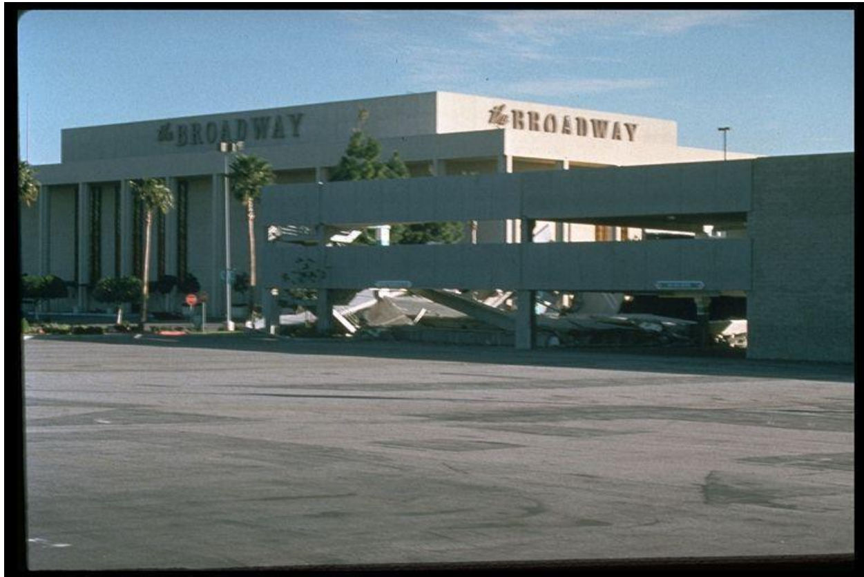
Figure 9–12. Image showing collapse of floors in the Northridge Fashion Center parking garage in the 1994 Northridge, California, earthquake.
