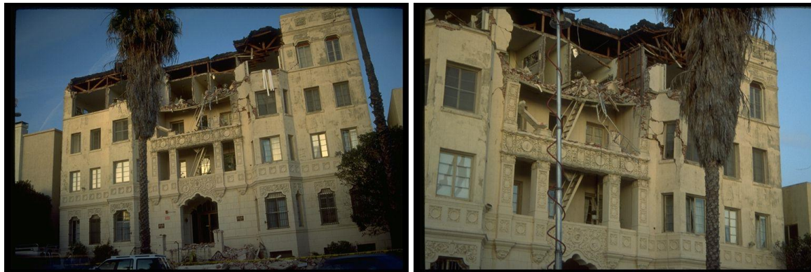
Figure 9–8. Image showing damage to four-story masonry building in Santa Monica in the 1994 Northridge, California, earthquake.
