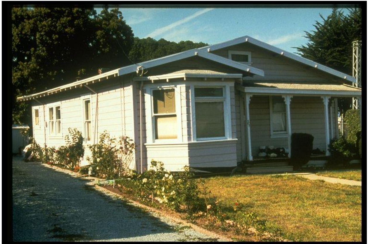
Figure 8–7. Image showing house with failed foundation in Watsonville in the 1989 Loma Prieta, California, earthquake.
