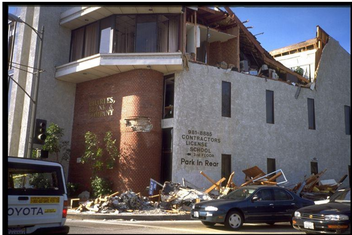
Figure 9–3. Image showing building components fallen onto off-ramp in the 1994 Northridge, California, earthquake.
