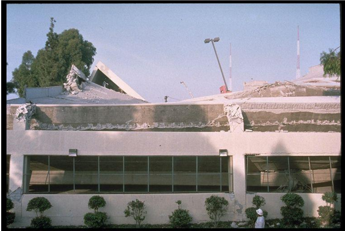
Figure 9–15. Image showing complete collapse of the Kaiser parking structure, Los Angeles, in the 1994 Northridge, California, earthquake.
