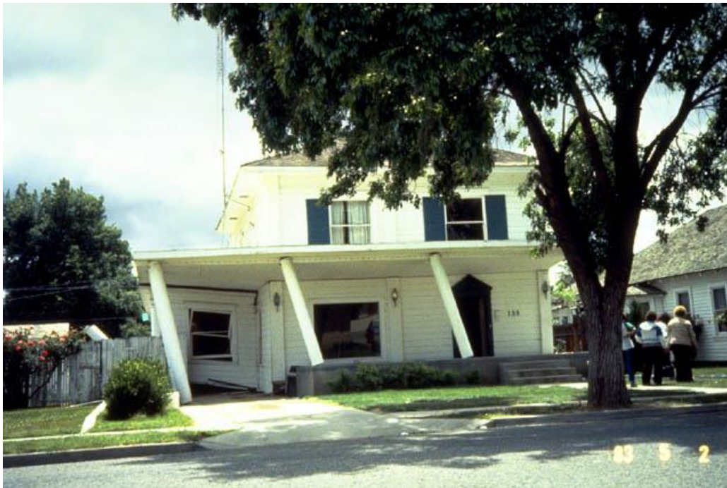
Figure 5-1. Image showing lateral displacement of two-story wood frame dwelling in the 1983 Coalinga, California, earthquake.
