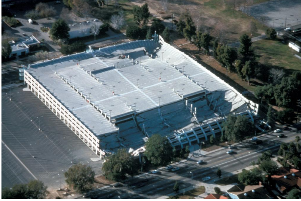
Figure 9. Example of a partially collapsed reinforced concrete structure: a parking structure at California State University, Northridge. Photo credit: P. Weigand. Permission for use granted per http://goo.gl/tmht1n .
