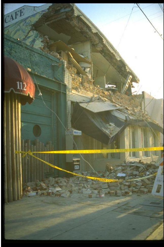
Figure 9-7. Image showing damage to two-story masonry building in Santa Monica in the 1994 Northridge, California, earthquake.
