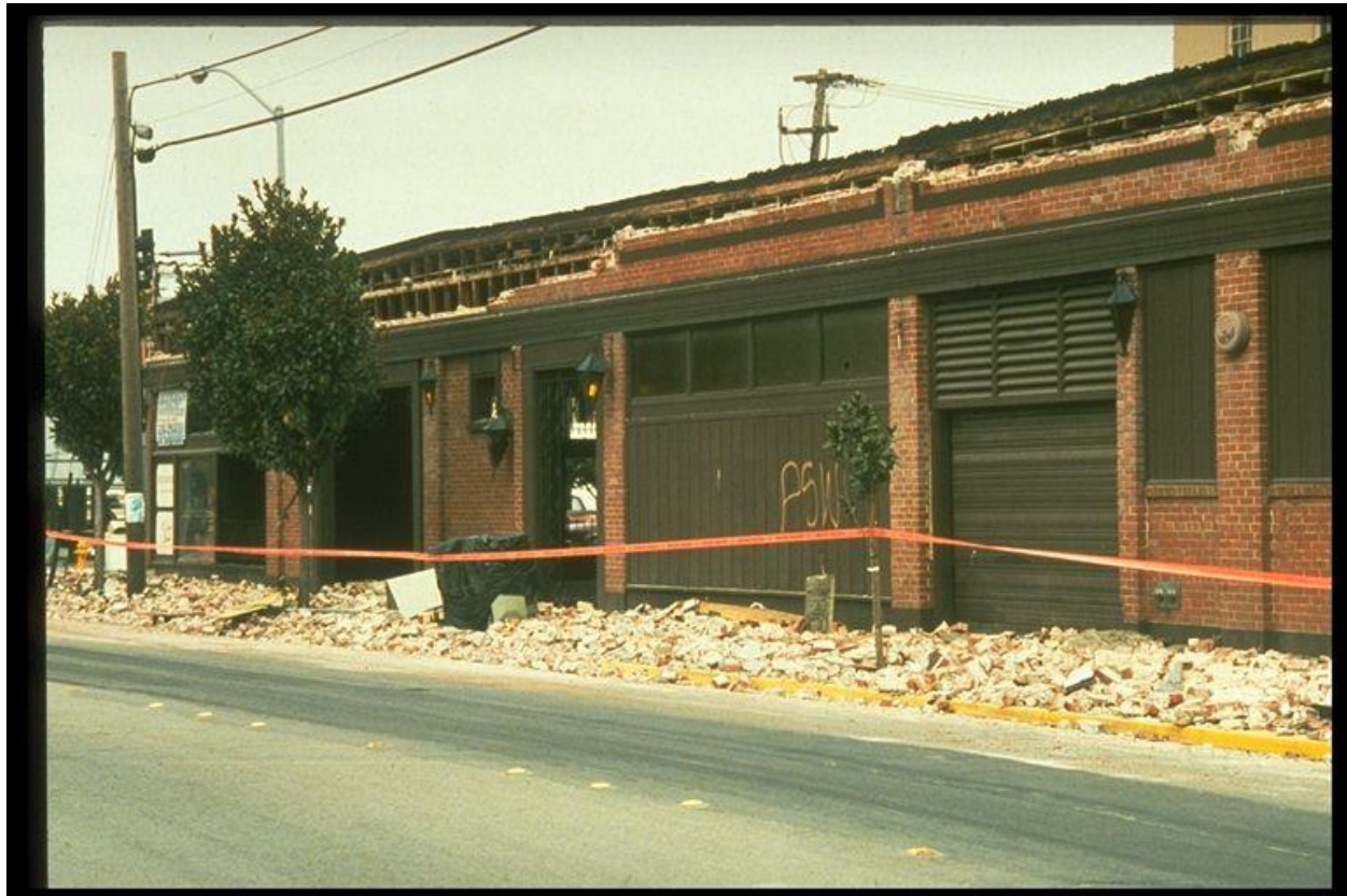
Figure 8-4. Image showing failed brick parapet fallen onto sidewalk in Watsonville in the 1989 Loma Prieta, California, earthquake.
