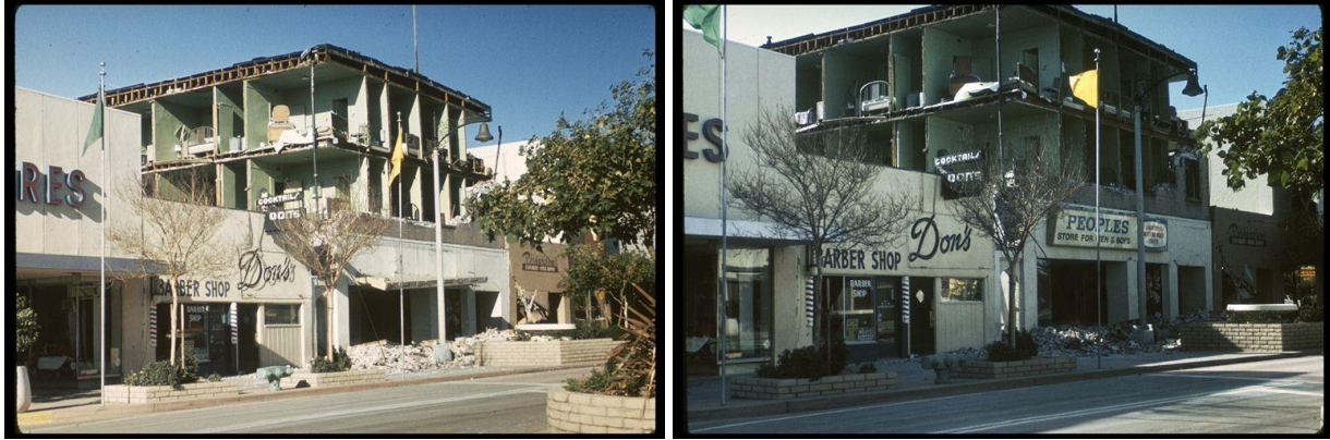
Figure 2-4. Images showing damage to apartments over retail space in the 1971 San Fernando, California, earthquake.
