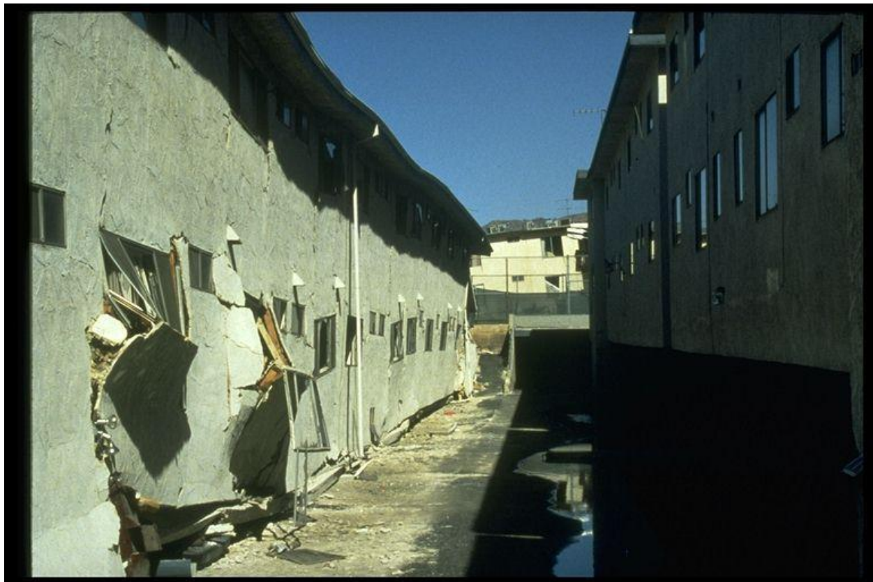
Figure 9-6. Image showing collapse of ground story at Northridge Meadows Apartments in the 1994 Northridge, California, earthquake.
