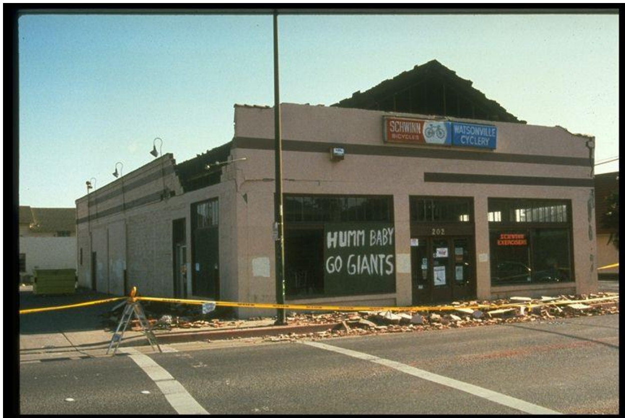
Figure 8–6. Image showing damaged bike store in Watsonville with failed parapet in the 1989 Loma Prieta, California, earthquake.
