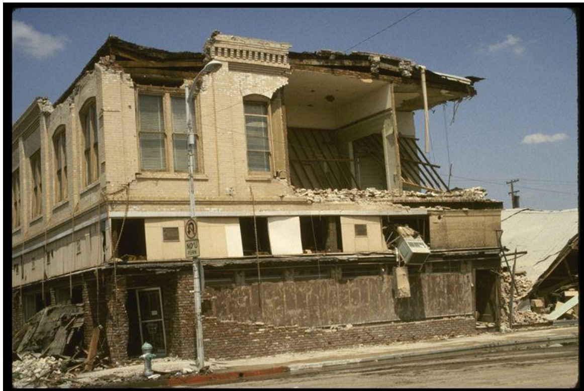
Figure 5-7. Image showing veneer fallen into first story of downtown building in the 1983 Coalinga, California, earthquake.
