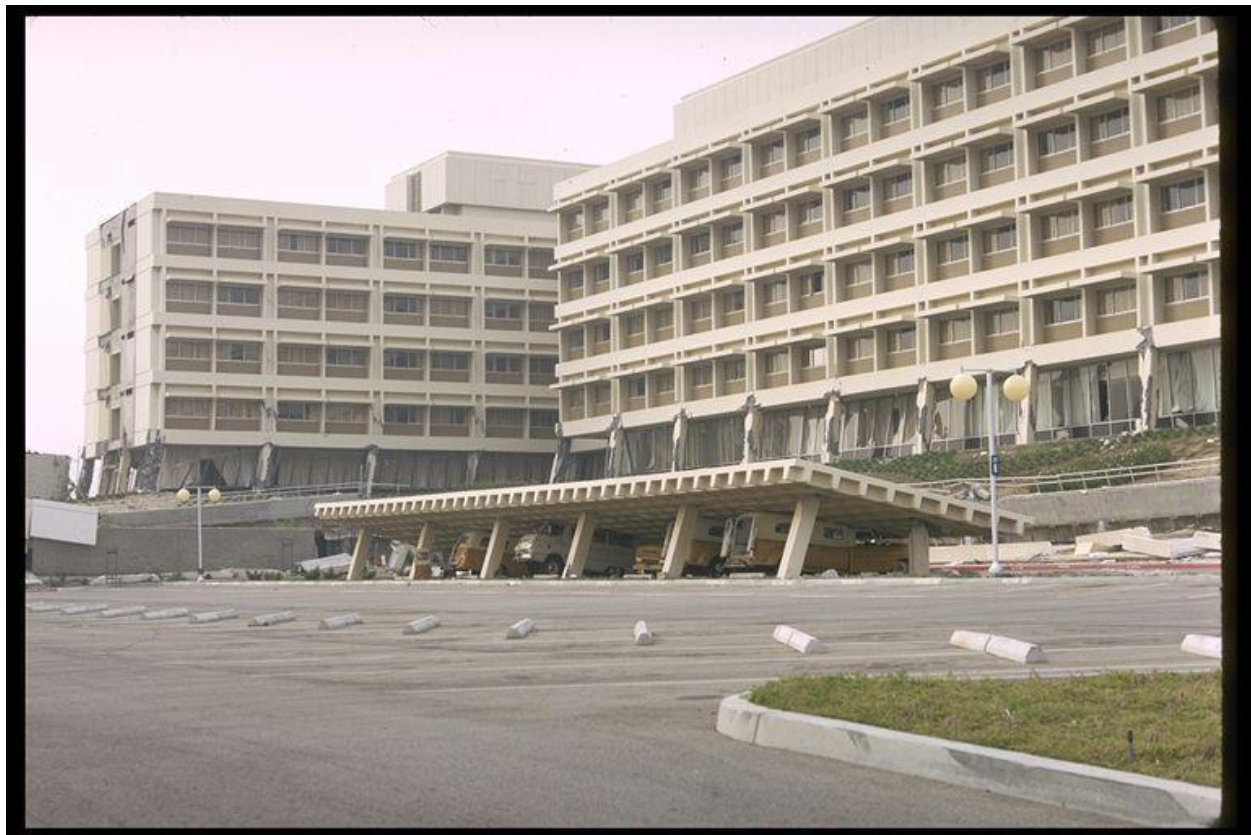
Figure 2-14. Image showing a collapsed ambulance garage at Olive View Hospital, Sylmar, in the 1971 San Fernando, California, earthquake.
