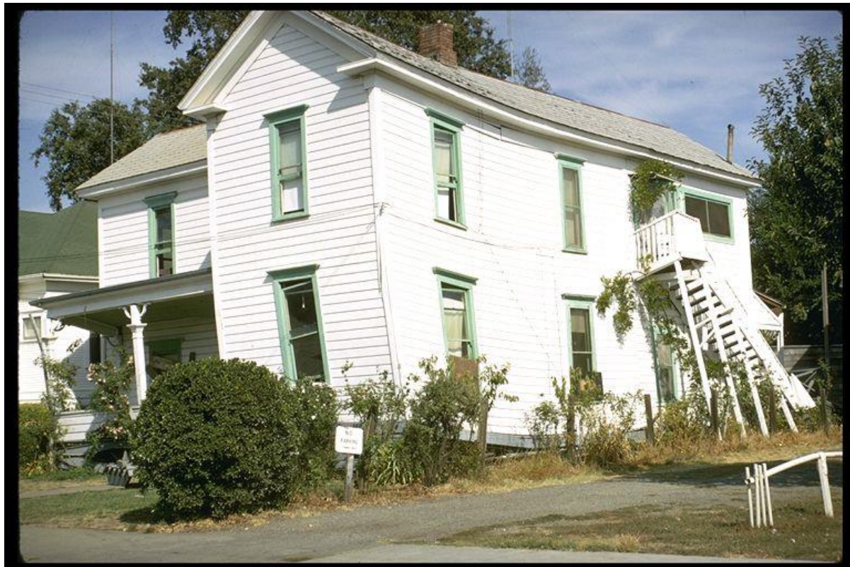
Figure 1-1. Image showing two-story wood frame house collapsed in the 1969 Santa Rosa, California, earthquake.
