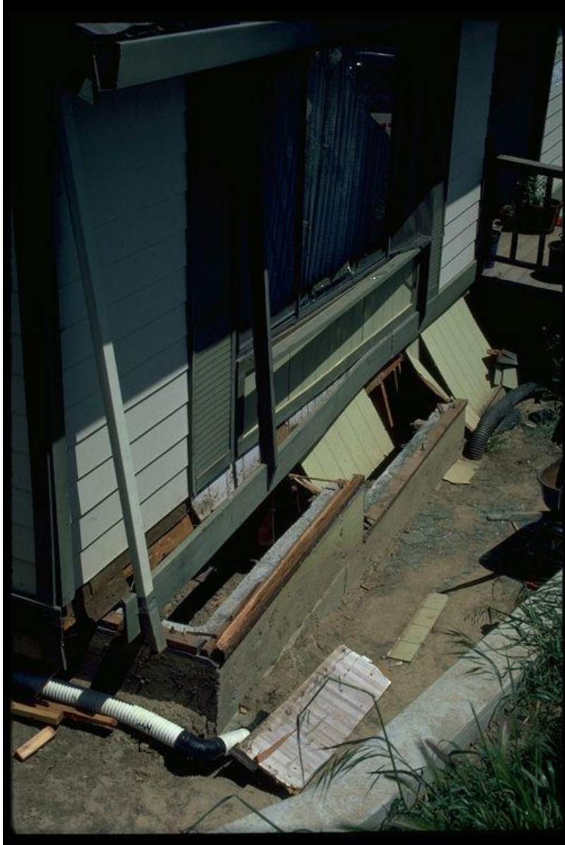
Figure 6-1. Image showing the most severely damaged dwelling in the 1984 Morgan Hill, California, earthquake.
