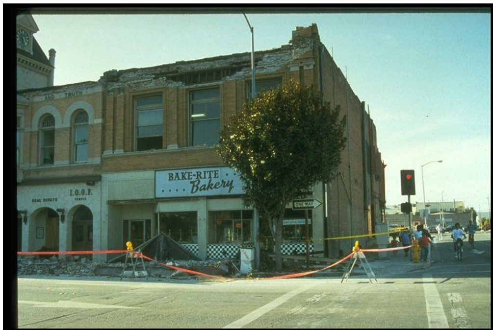
Figure 8-2. Image showing parapet and wall failures in Watsonville in the 1989 Loma Prieta, California, earthquake.
