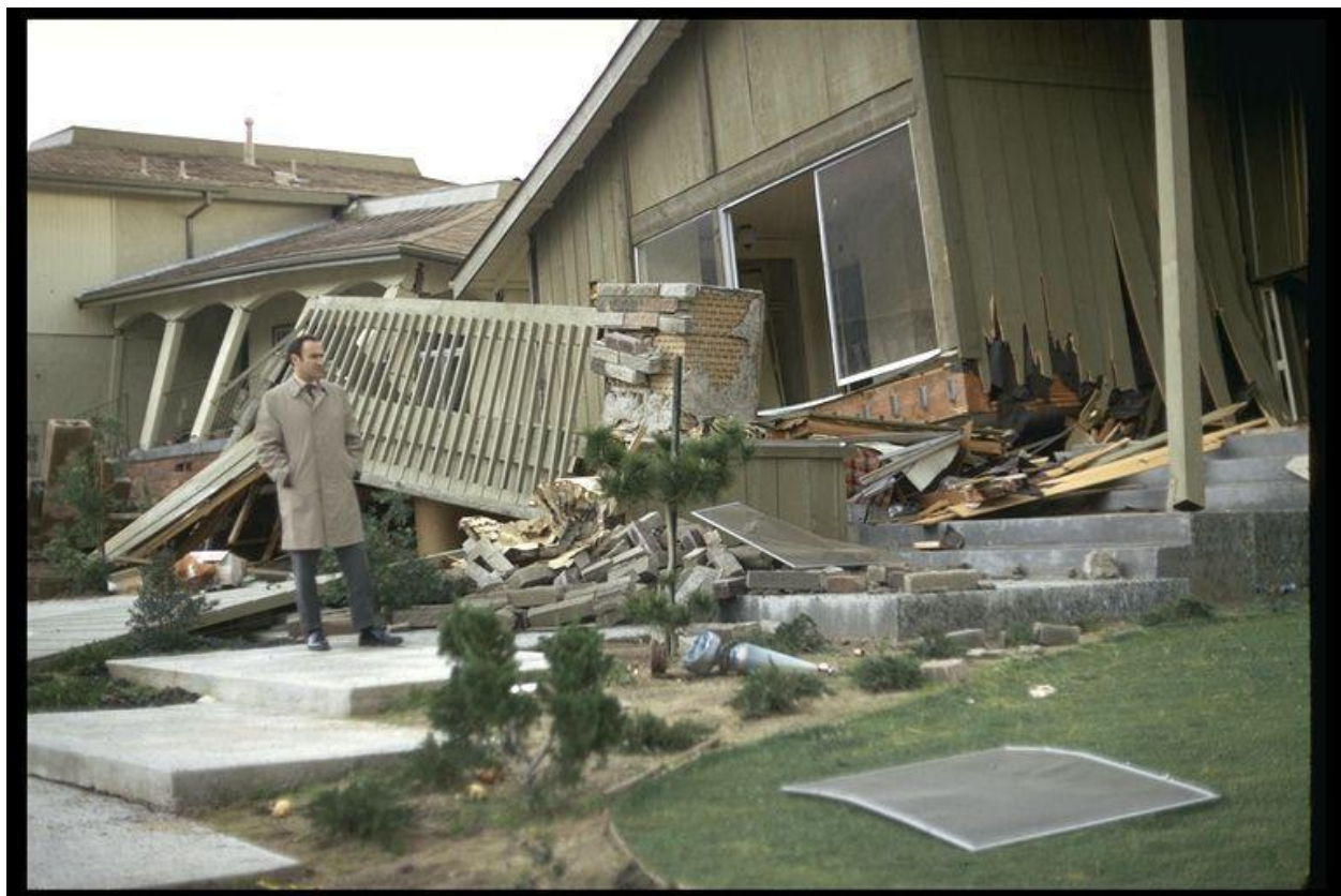
Figure 2–18. Image showing soft-story failure in a wood frame house in the 1971 San Fernando, California, earthquake.
