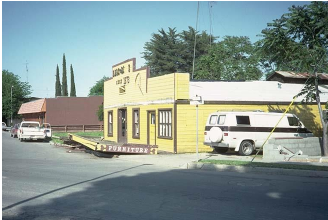
Figure 5-5. Image showing a heavy wooden overhang fallen onto sidewalk in the 1983 Coalinga, California, earthquake.
