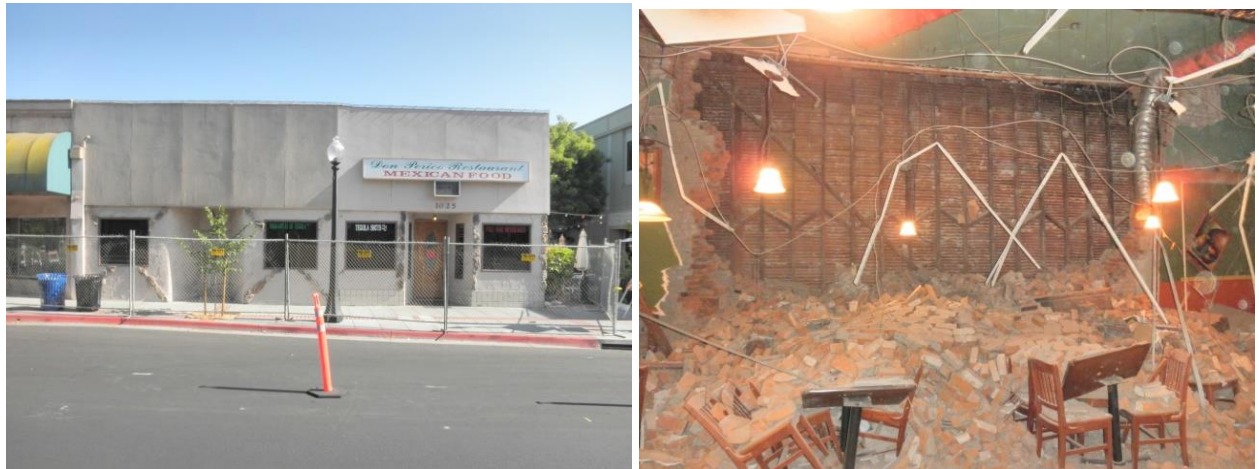
Figure 11–1. Image showing damage to Don Perico's Restaurant in Napa in the 2014 South Napa, California, earthquake.
