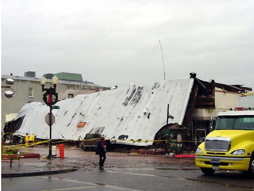
Figure 10–1. Image showing collapsed building from intersection of 12th and Park Streets in Paso Robles in the 2003 San Simeon, California, earthquake.
