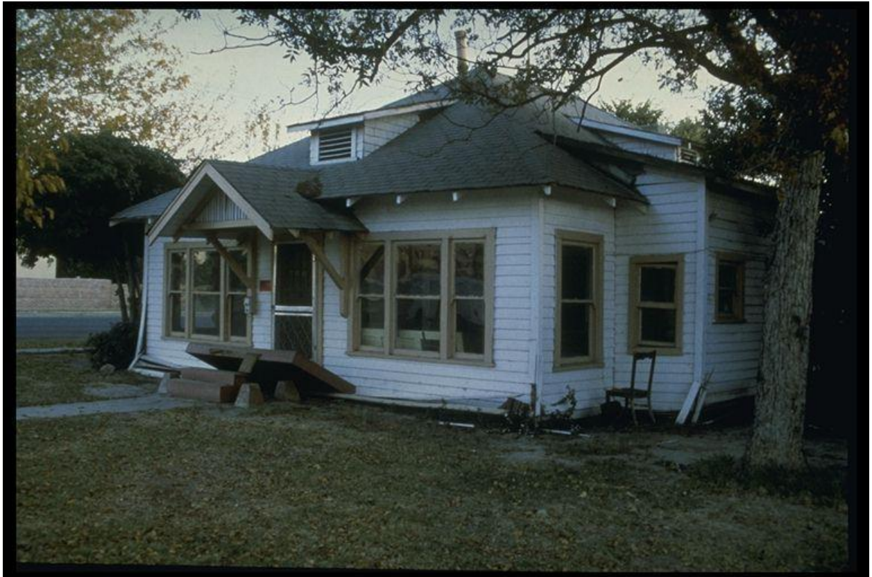
Figure 3–3. Image showing cripple wall collapse on a wood frame house in the 1979 Imperial Valley, California, earthquake.
