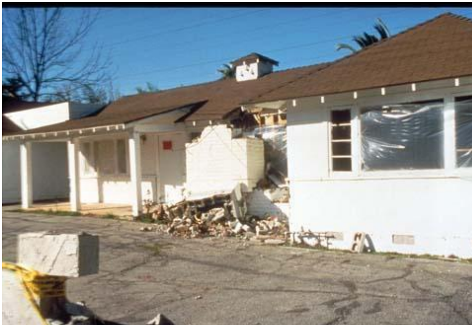
Figure 9–9. Image showing collapsed unreinforced chimney in the 1994 Northridge, California, earthquake.
