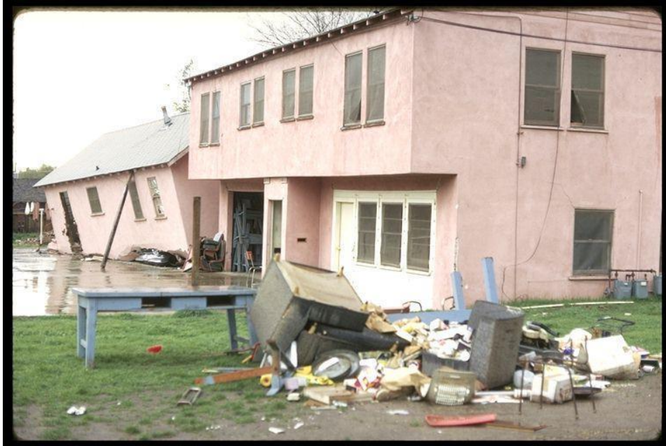
Figure 2-7. Images showing soft-story failure in the 1971 San Fernando, California, earthquake.
