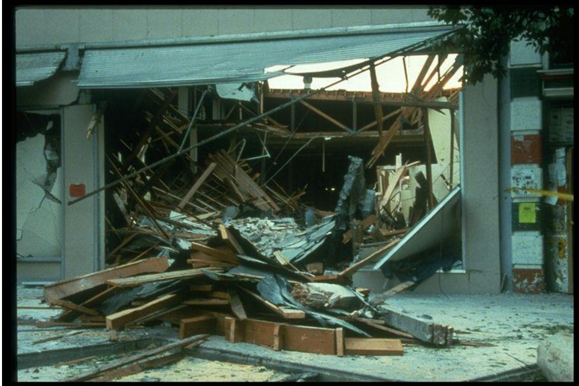
Figure 8–14. Image showing interior structural failure in a department store in Santa Cruz in the 1989 Loma Prieta, California, earthquake.
