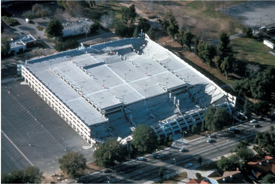
Figure 9–11. Photograph from the 1994 Northridge, California, earthquake. Image is taken from Earth Science World Image Bank ( http://goo.gl/gdASRH ), which describes it as follows: “California State University, Northridge parking structure that partially collapsed during the 1994 earthquake. Scientists believe it was the lack of shear walls, being precast, and lack of extra steel reinforcements in vertical columns that led to the damage seen here. This is 5km northeast of the epicenter.” Photo by P.W. Weigand. Copyright California State University, Northridge, Geology Department. Permission granted per http://goo.gl/tmht1n .
