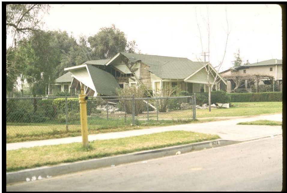
Figure 2-1. Image showing damage to a wood frame house in the 1971 San Fernando, California, earthquake.
