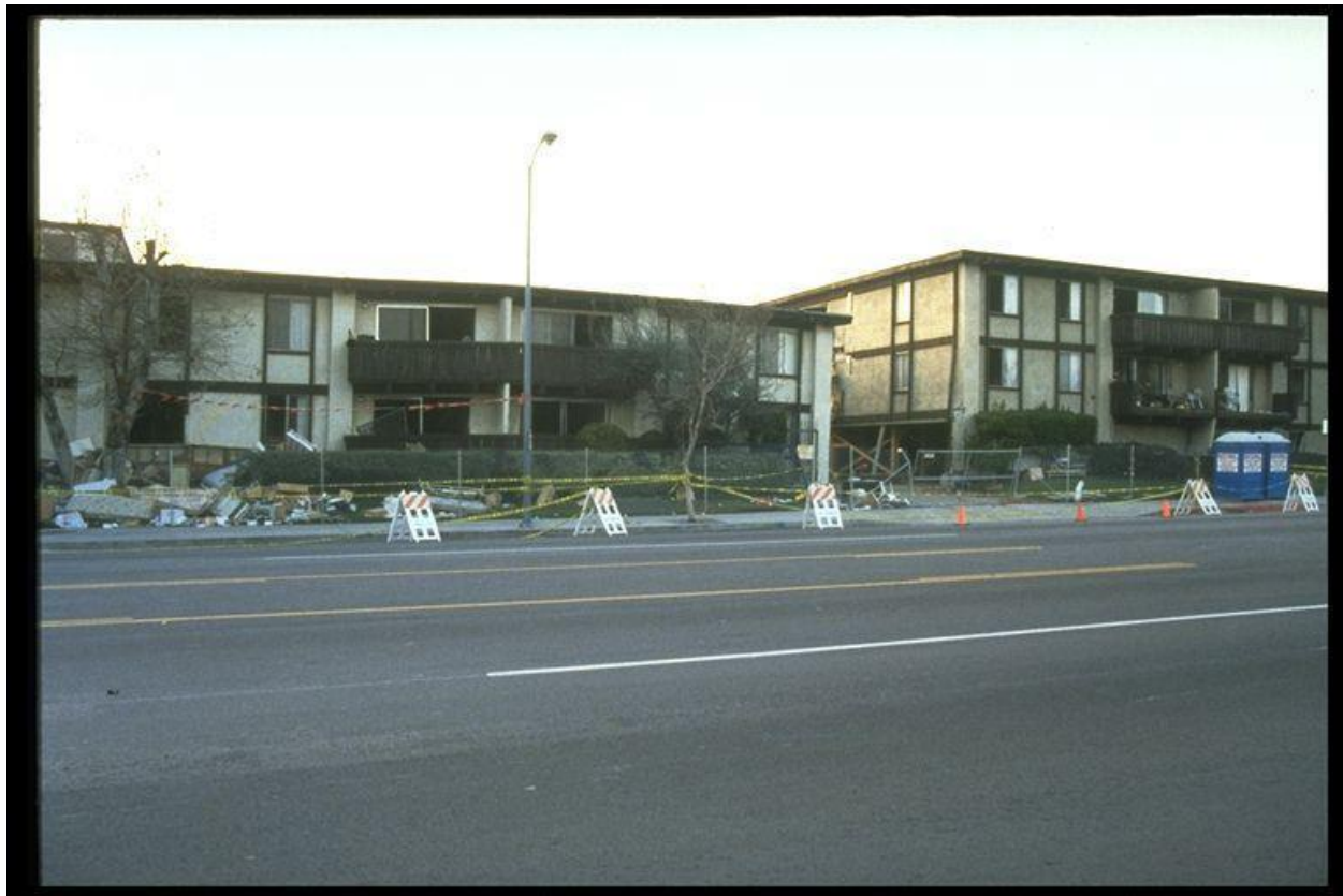
Figure 9-4. Image showing collapse of ground story at Northridge Meadows Apartments in the 1994 Northridge, California, earthquake.
