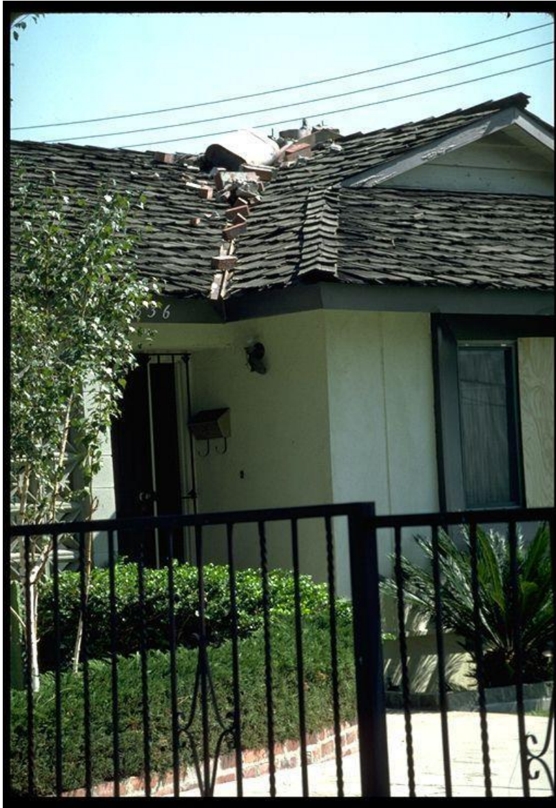
Figure 7-1. Image showing damage to roof from collapsed chimney in the 1987 Whittier Narrows, California, earthquake.
