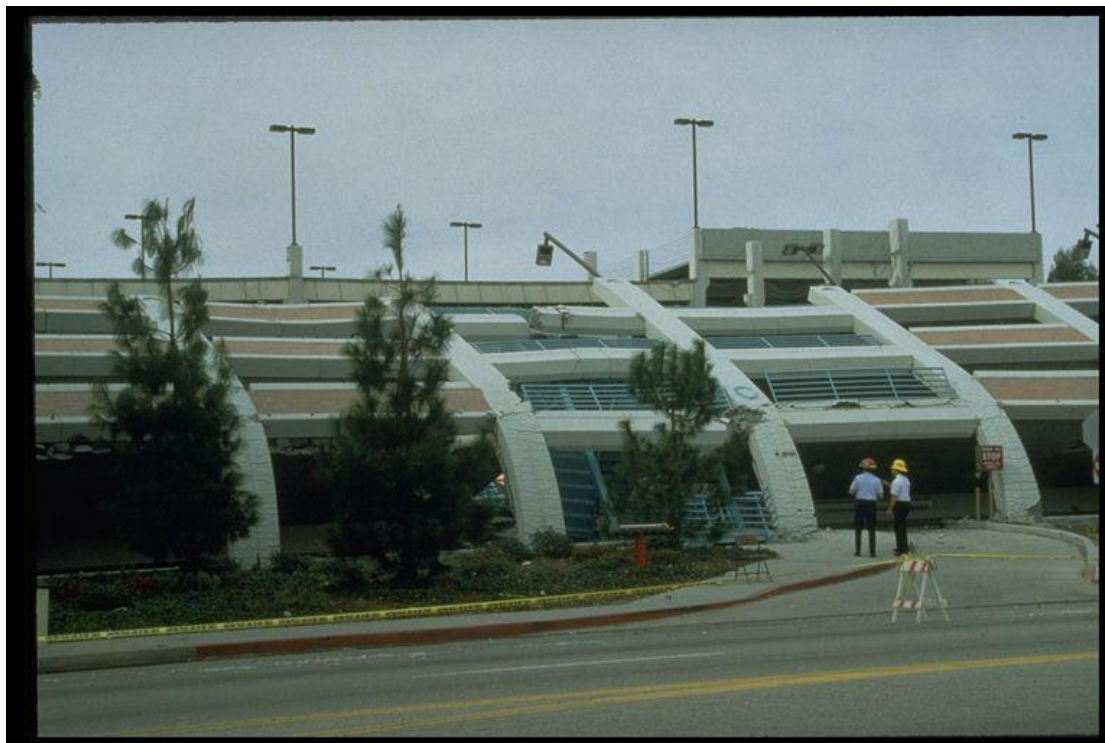
Figure 9–10. Image showing collapse of a parking structure on the California State University, Northridge, campus in the 1994 Northridge, California, earthquake.
