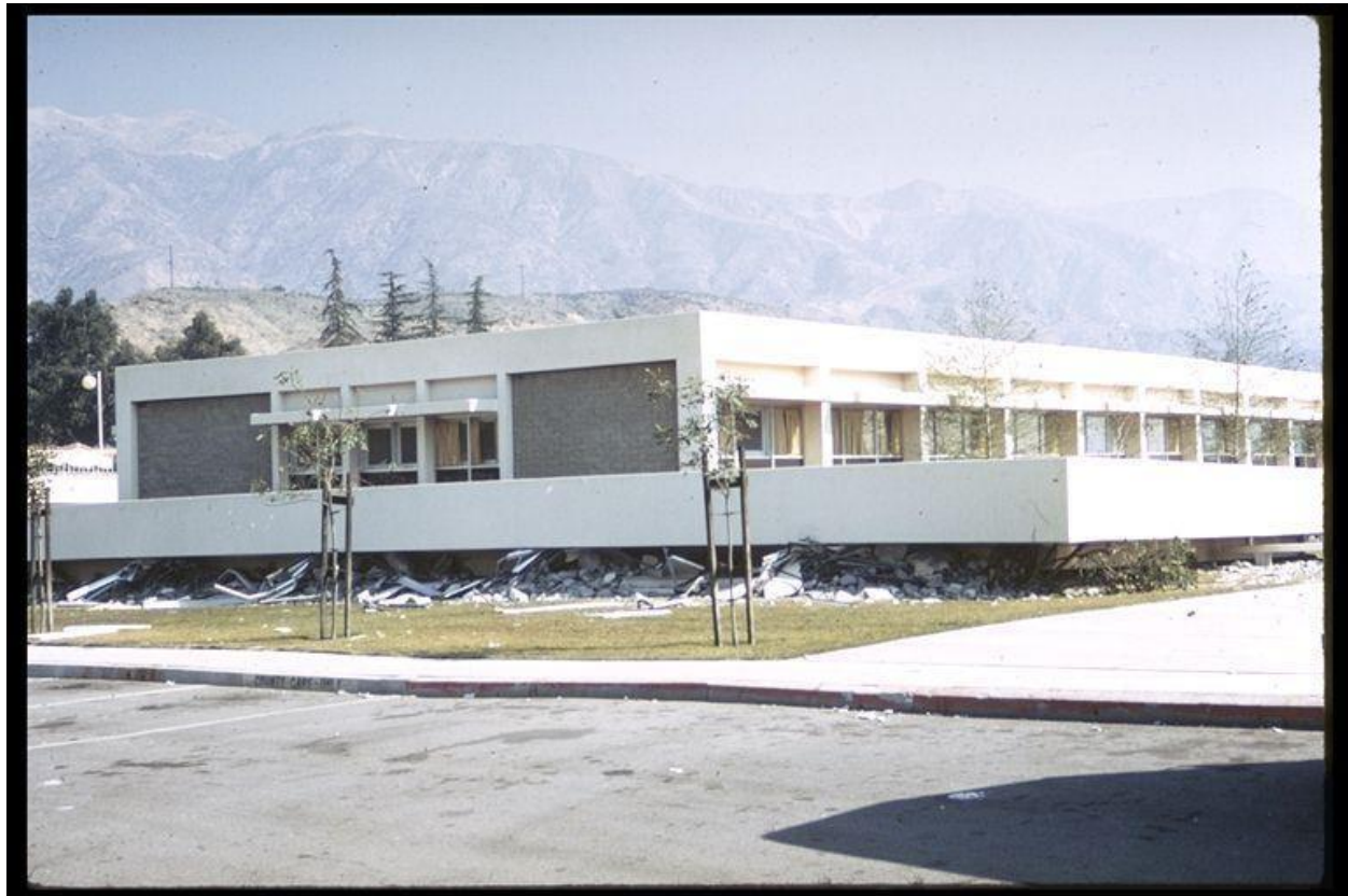
Figure 2–16. Image showing first story collapse of Psychiatric Building at Olive View Hospital, Sylmar, in the 1971 San Fernando, California, earthquake.
