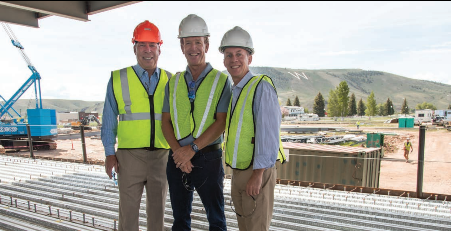
From left, Western Colorado University President Greg Salsbury, donor Paul M. Rady and former CU Engineering Dean Bobby Braun tour the new Paul M. Rady School of Computer Science & Engineering building in Gunnison during construction in June 2019.
