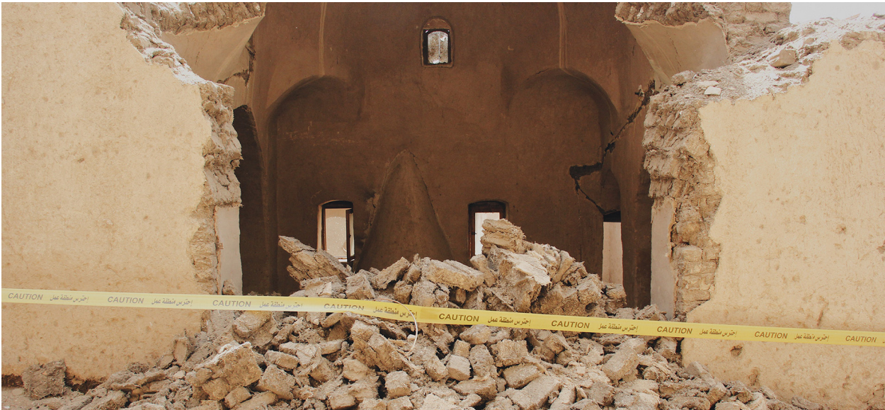
Decaying buildings awaiting restoration in New Gouna. Samir.
