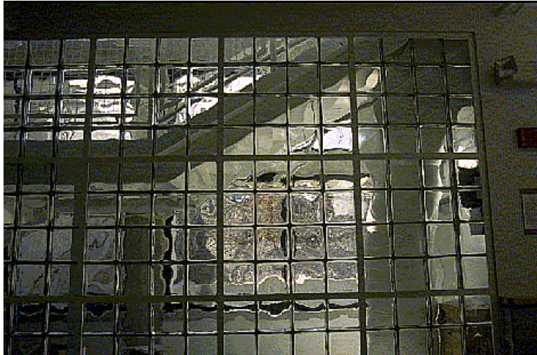
Figure 8.35. Square glass blocks provide fire safety and allow natural light to illuminate a basement laboratory plaza in the ITLL.
