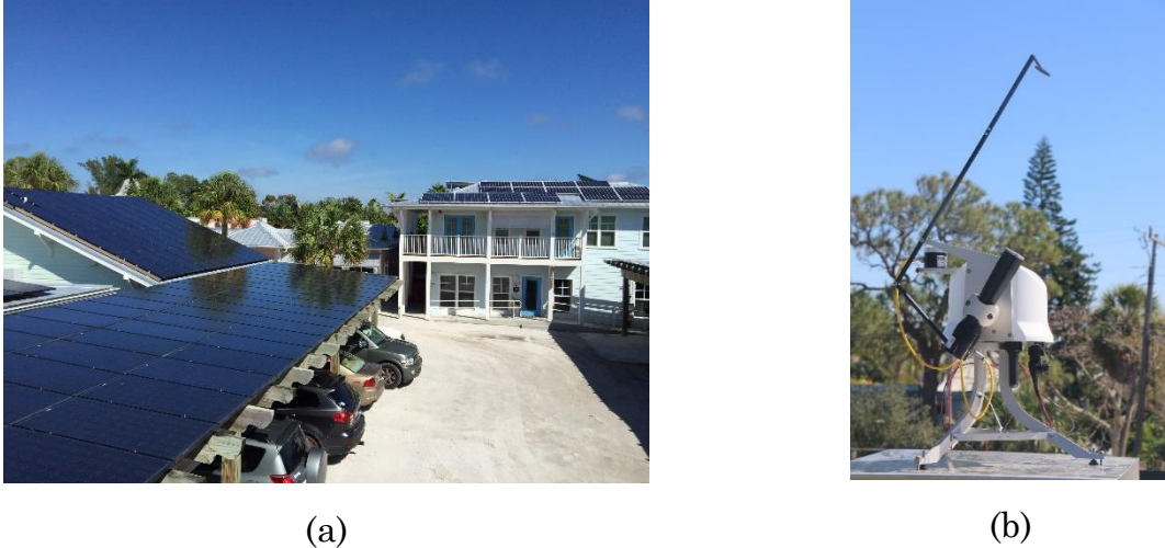
Figure 3.1 Photos of the roof-top PV panels (a) and the weather station (b).
