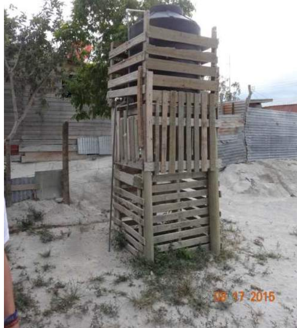
Image 8: The water source for the community dining hall is unsecured and easily accessible, making it vulnerable to vandalism and sabotage.
