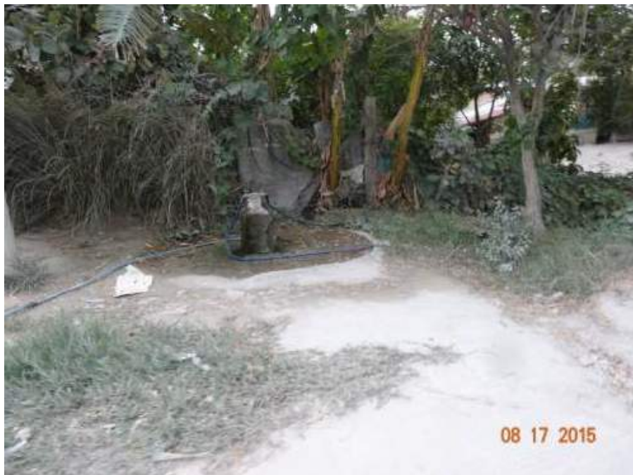
Image 9: Water distribution system consisting of hoses and hose bibs.
