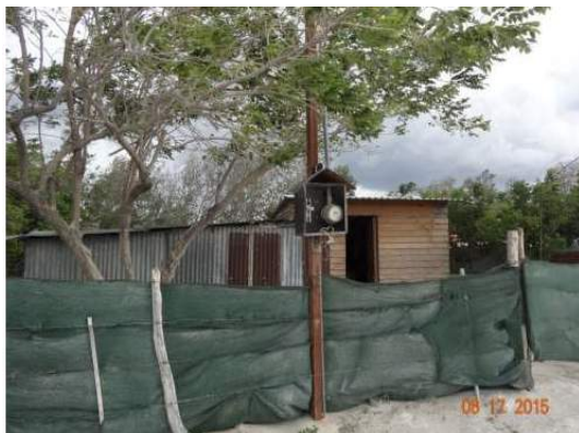
Image 14: Open meter box and exposed wires.
